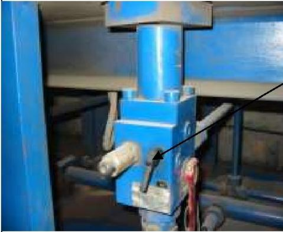
ARROW IN THE PICTURE IS SHOWING DRAIN VALVE FIGURE- 3
