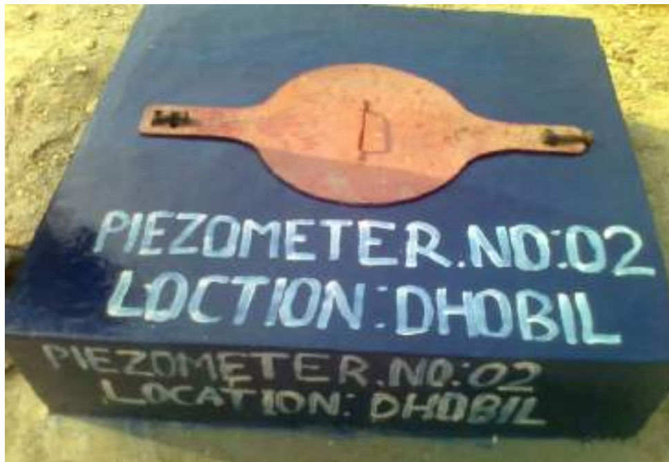
2. Piezometer at Dhobil Village
