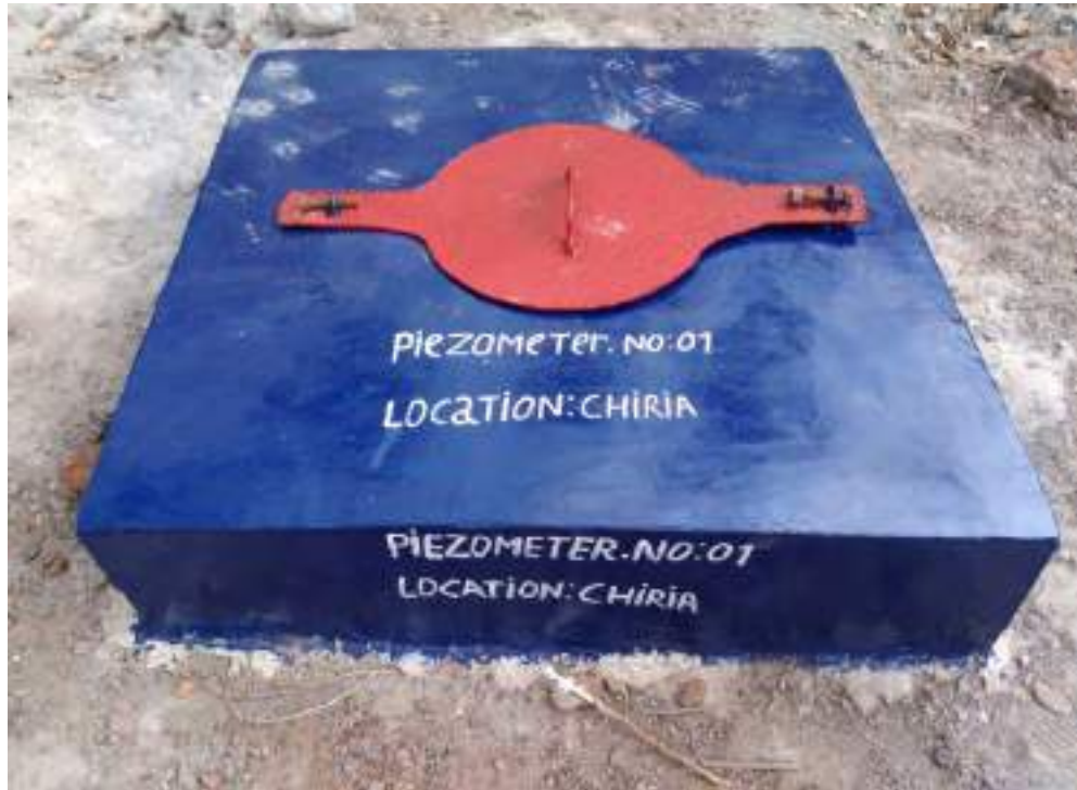
1. Piezometer at Chiria Village
